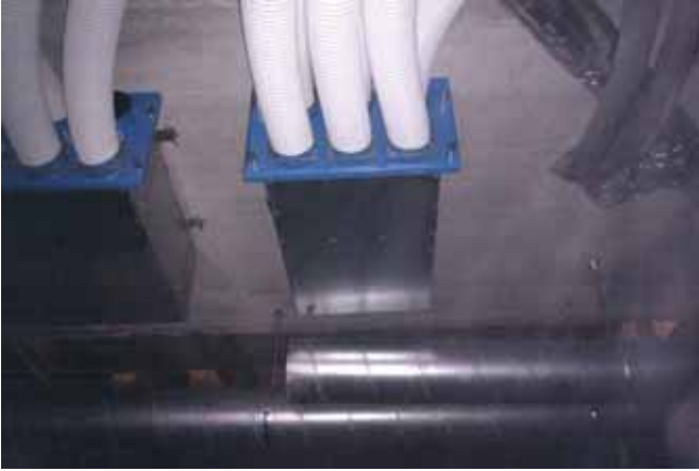
23.09.2010 Air handling ductwork, Octopus system installed
