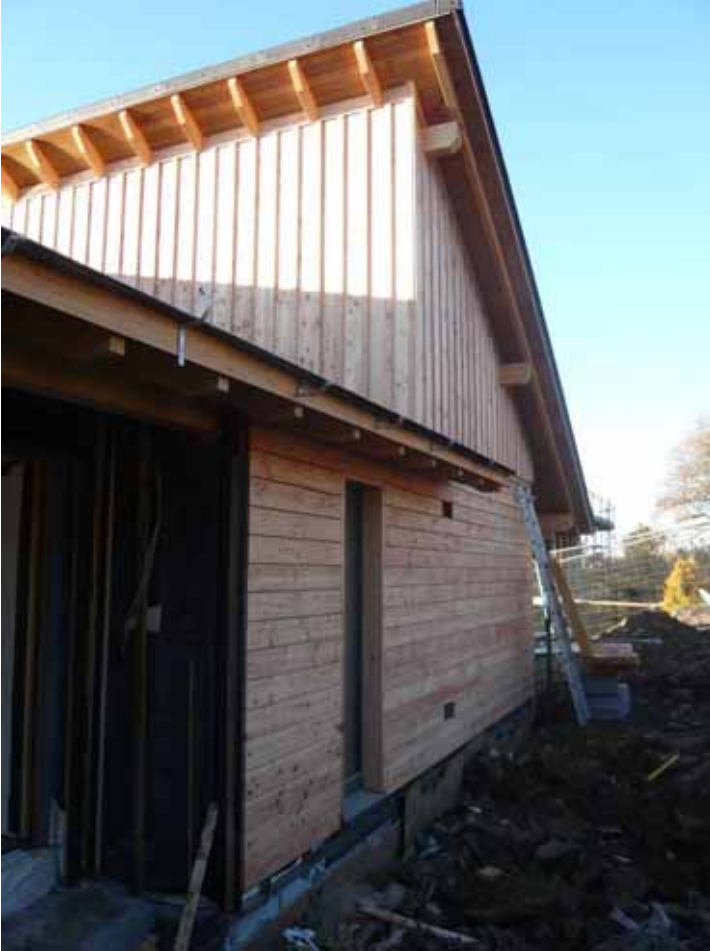
08.12.2010 Cladding continues - but more insulation to be fitted at plinth before cladding completes
