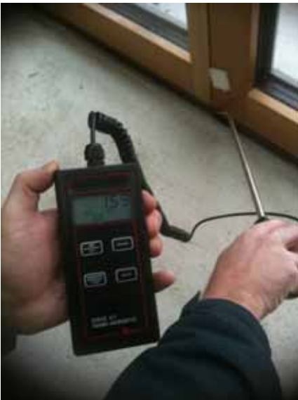
30.11.2010 Finding the leak is nearly as good as fixing it!
